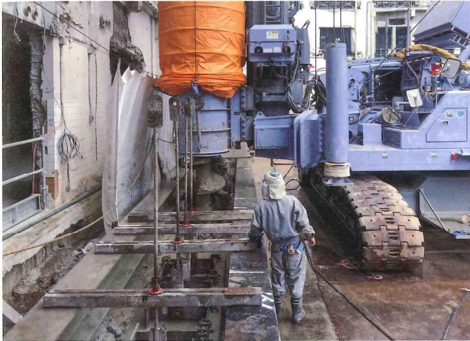
保存棟際SMW施工状況。 | SMW construction on the edge of the preserved building.
